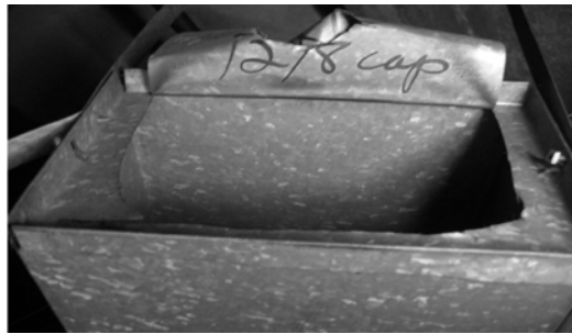
Figure 4.1: A service opening left open by a duct cleaner.
